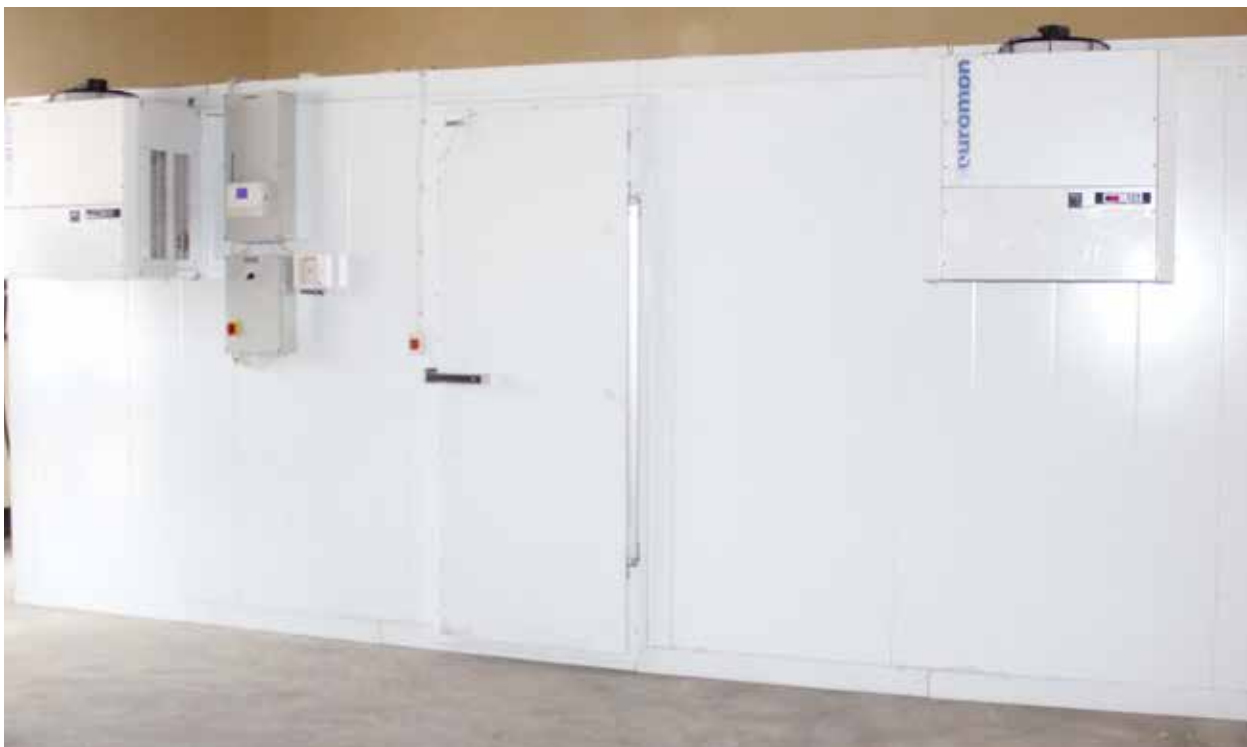
The newly installed cold room in Chinsali, Muchinga Province
