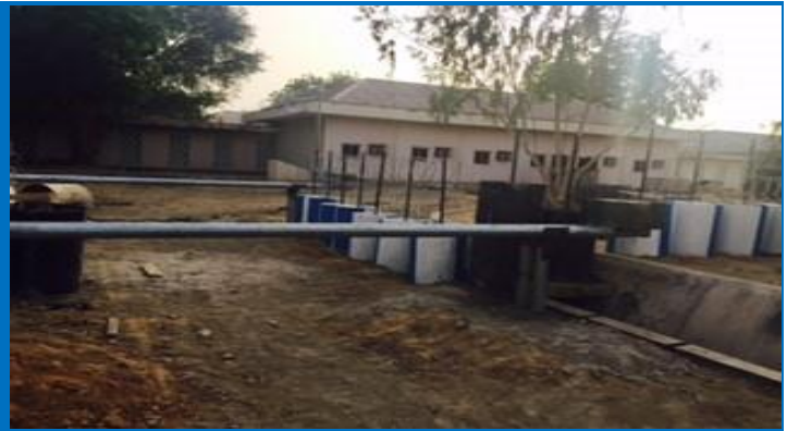
Work in progress on the Borno State Public Health Emergency Operations Centre in Maiduguri. (Photo: WHO)
